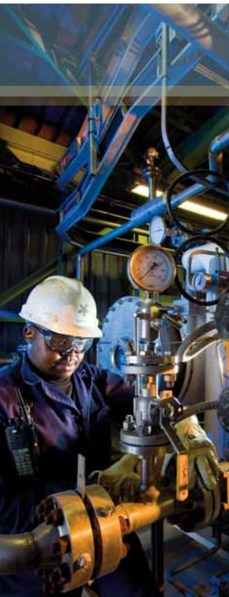
Pule Letuba , process controller at the Secunda water recycling project, checks an ozone generator unit
